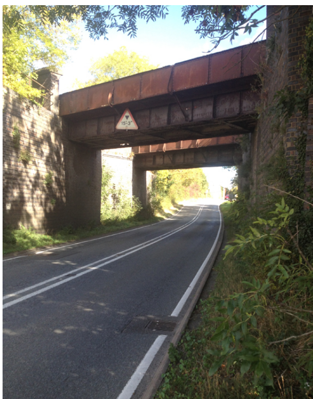
Figure 1. The bridge of the former Great Central Railway over the A421 road, just south of the former Fimmere station in Buckinghamshire, England (photographed in October 2018).
